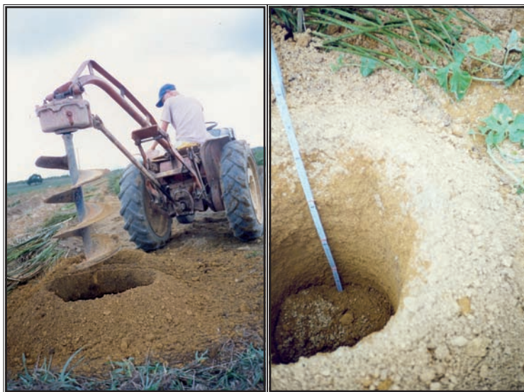
Figure 11. Earth Auger, or soil drill, with a diameter of 18” employed to make planting holes.
